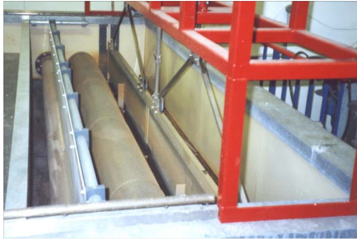
(a) Weir gate and manifold area
