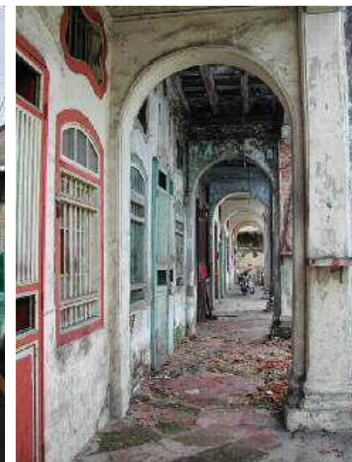
(c) & (d) Poor buildings waiting for renovation
