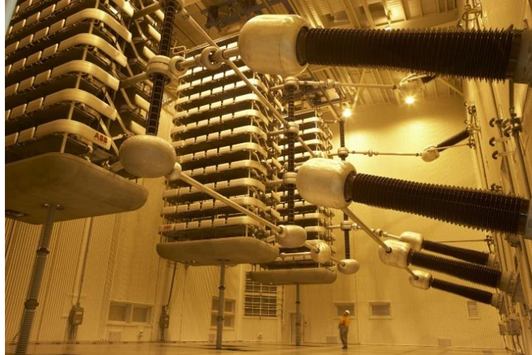
Fig. 2. 25. LCC transformer wall bushings inside the valve hall [126].
