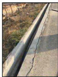
Longitudinal crack on landfill berm surface
