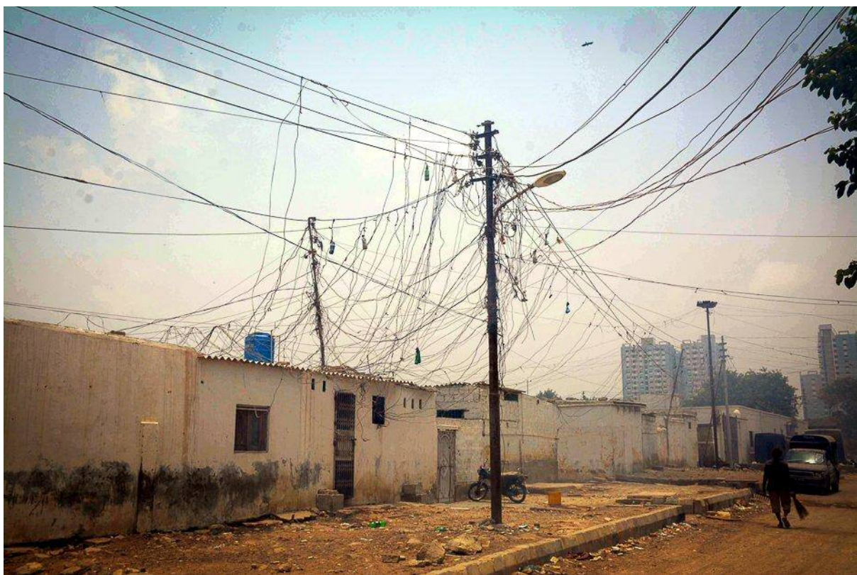
Figure 7.1 The Network of Illegal Connections
