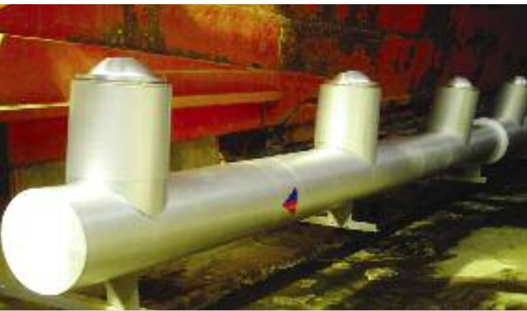
Figure 7. Desiccated air distribution nozzles
