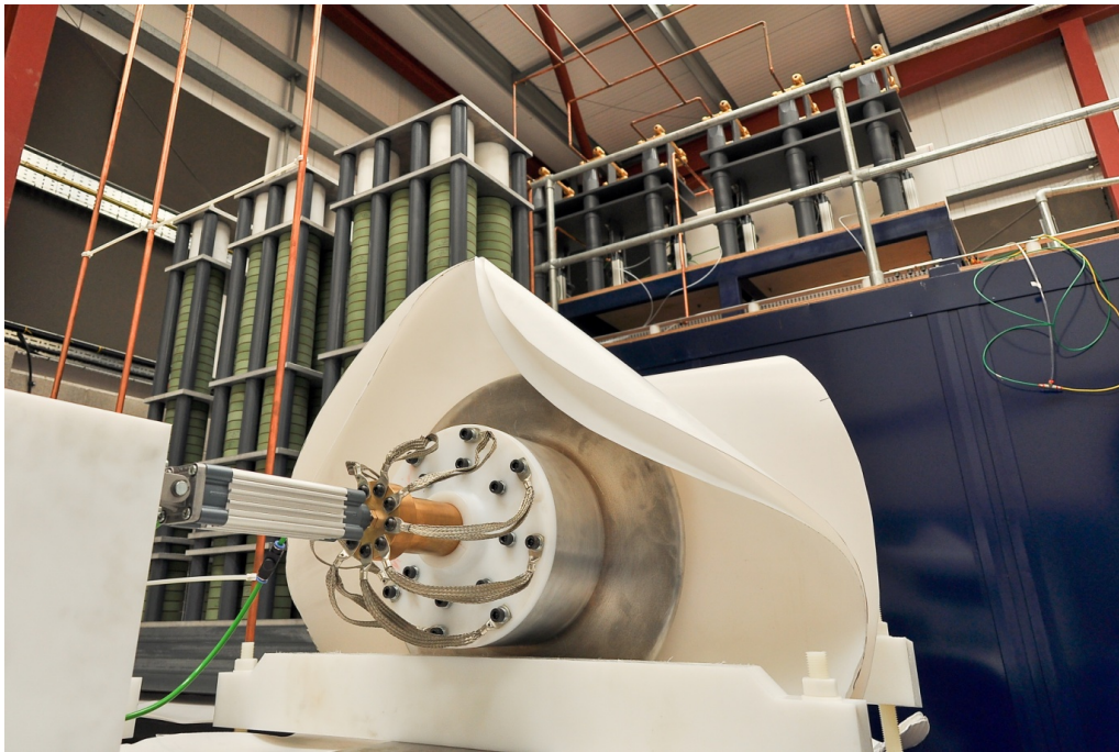
Figure 50 – Pneumatically operated high current spark gap switch
