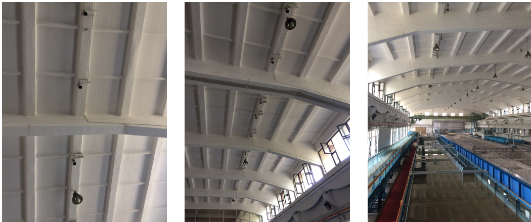
Figure 4.6: PTV camera system installed above flume
