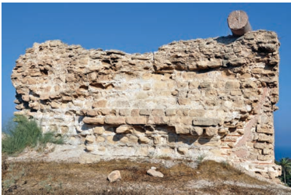
Figure 19.89. The southern block of Wall WW from the east, showing the Phase 2 (Byzantine) wall overlain by Phase 1 (Umayyad/Abbasid) rebuilding (photo Denys Pringle 2012)
