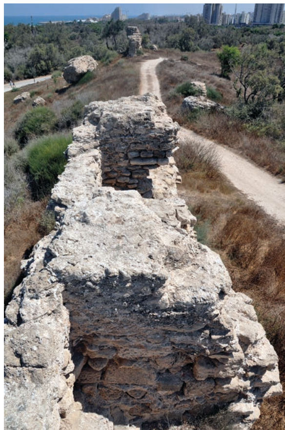
Figure 19.74. Curtain wall to the north of Tower K, looking north toward Grid 34 along the present wall head (photo Denys Pringle 2012)
