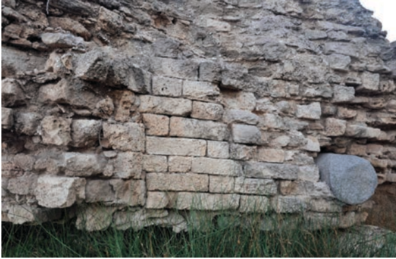
Figure 19.85. Triangular Turret VV (upside down), showing the bonding between the northeast face (right) and the curtain wall (left) (photo Denys Pringle 2012)
