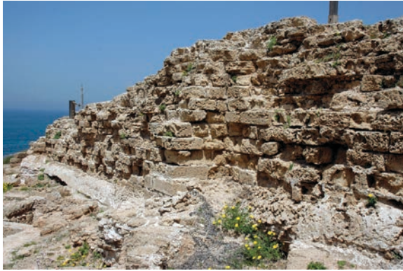
Figure 19.158. Arsuf (Apollonia): Umayyad town wall with external buttresses as it appears on the south (photo Denys Pringle 2009)
