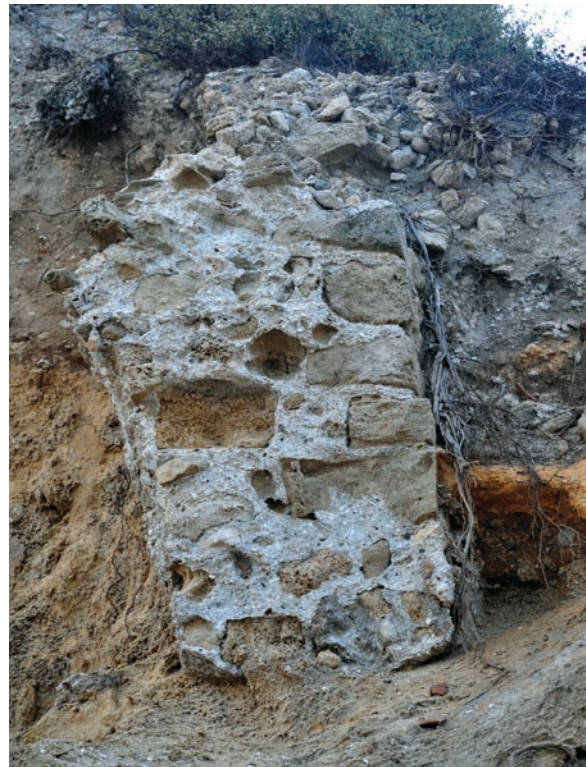
Figure 19.40. The section through a possible outer Wall JJ6 visible in the eroded cliff south of Tower JJ5 (photo Denys Pringle 2012)
