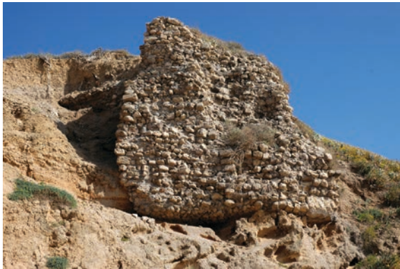
Figure 19.38. The foundation of Tower JJ5, viewed from the beach below (photo Denys Pringle 2009)
