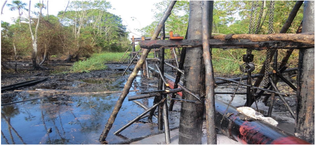
Figure 2: View of the North Peruvian Pipeline after the completion of repairs to the 2014 rupture that affected Cuninico. Its poor condition is obvious from this photo (Figure 2 provided by a Cuninico resident given to them by a Petroperu engineer and used with their permission, Summer 2014).
