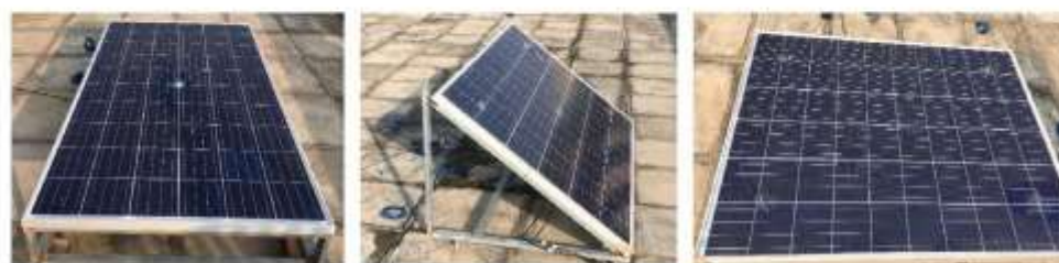
a. Horizontally-mounted PV roof b. Tilted PV roof c. Firmly-attached PV roof
