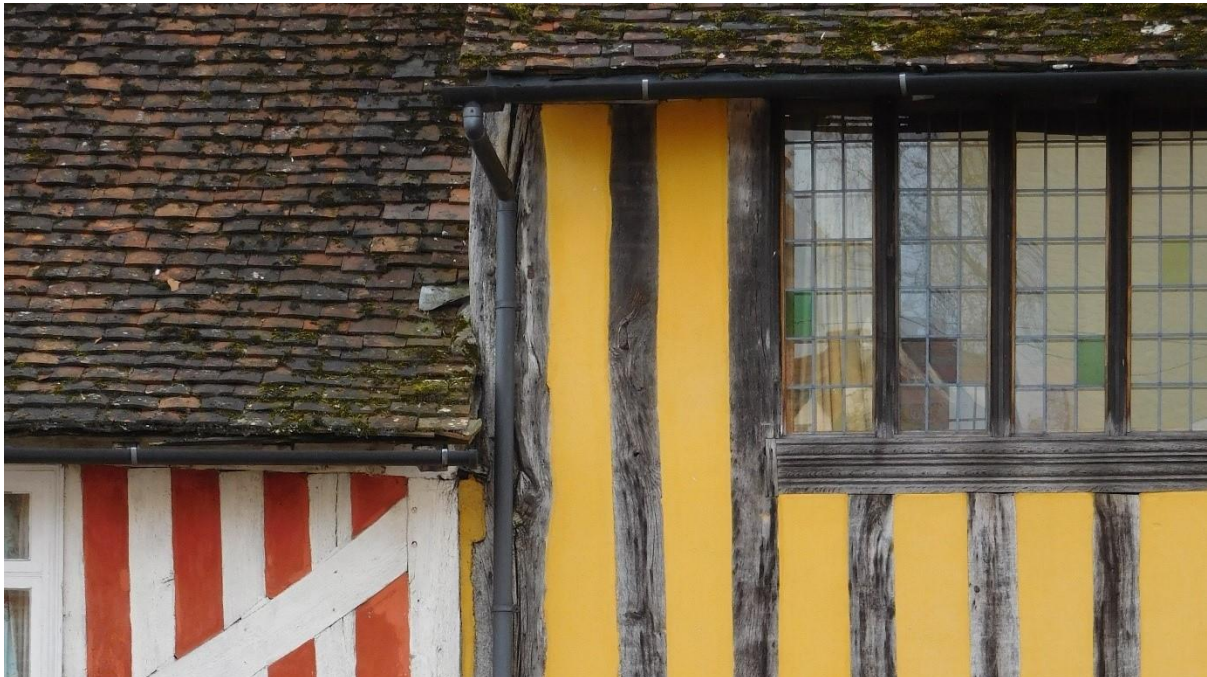
Figure 1. C15th timber framing, The Manor House (left) and 53 Church Street (right), Lavenham, Suffolk, © Whitman
