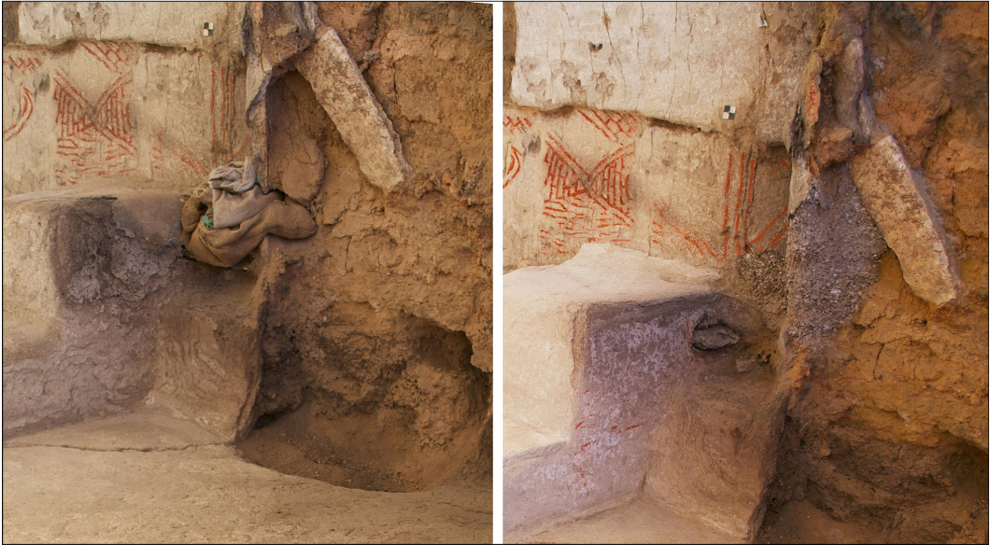
Figure 14.5. (left): Building 80, F.5014 showing sandbags stabilizing a falling plaster column; (right): replacement of the column with a perlite structure.
