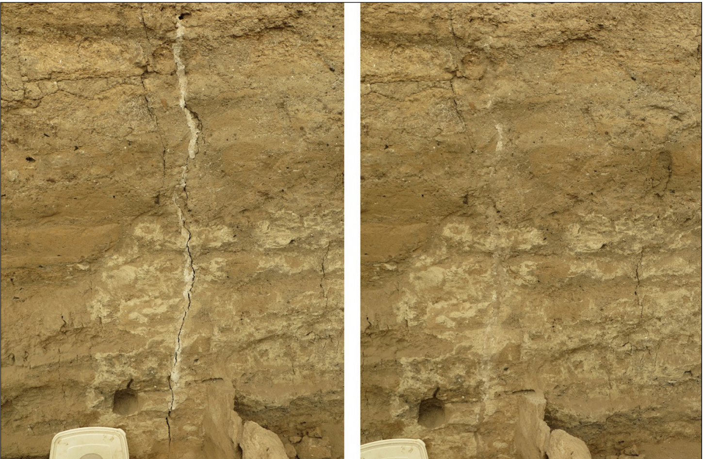
Figure 14.4. (left): Building 119, F.220 shows a failing lime fill and expanding crack; (right): the gap after removal of the lime fill and replacement with perlite.
