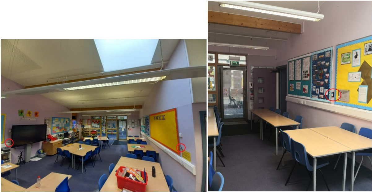
Figure 5: T/RH and CO 2 sensors in School A - Year 6
