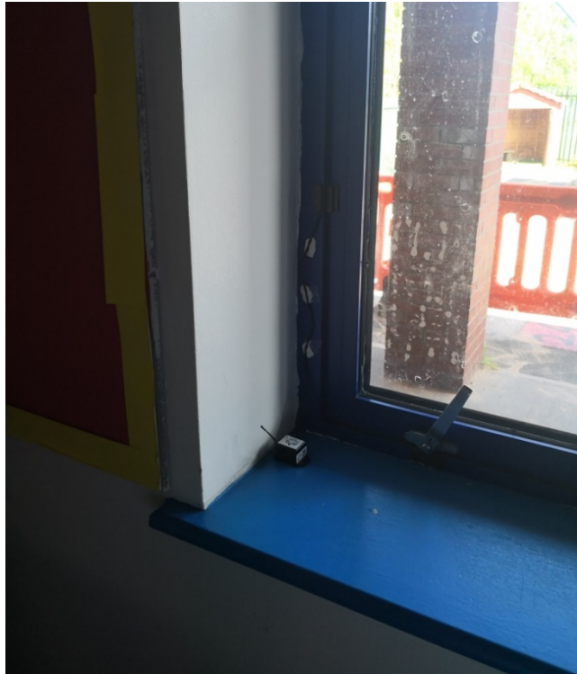
Figure 9: Window open/closed status installed sensor in School B
