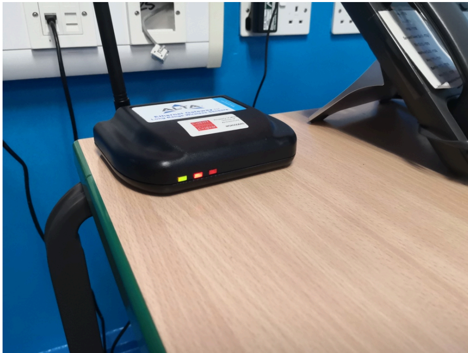
Figure 10: The gateway for receiving and transmitting the monitoring data
