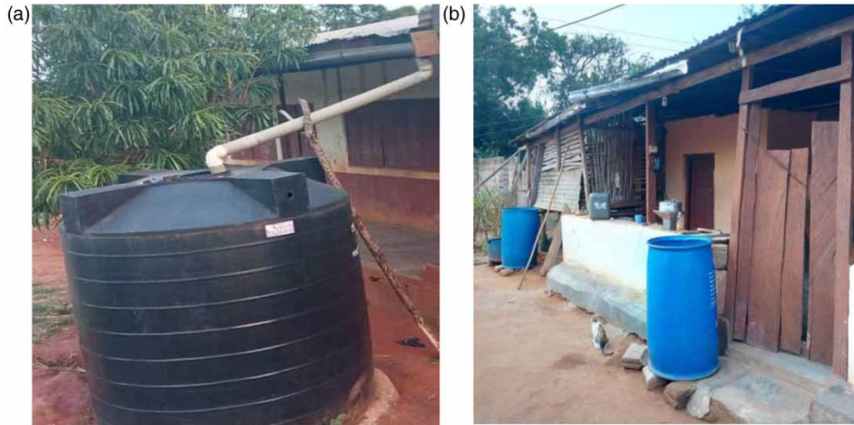
Plastic storage tanks
