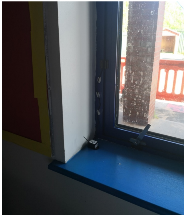
Window open/closed status installed sensor in School B
