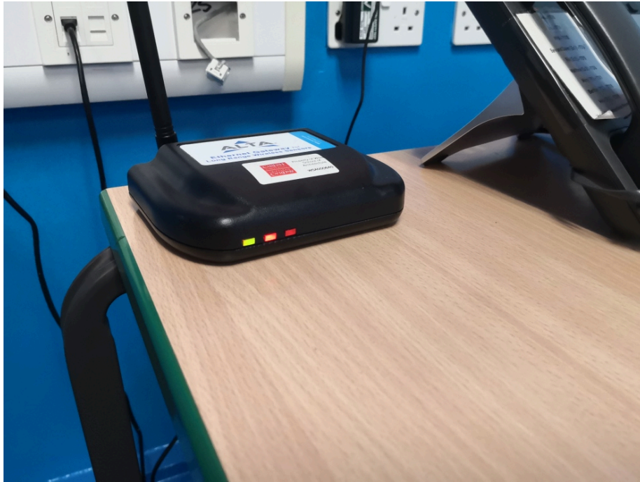
The gateway for receiving and transmitting the monitoring data
