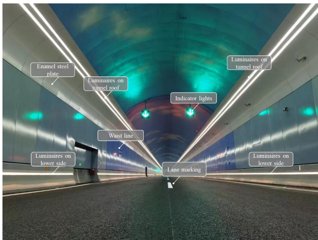
583 584 Fig.14 The view of the interior environment in Boao Tunnel under operation
