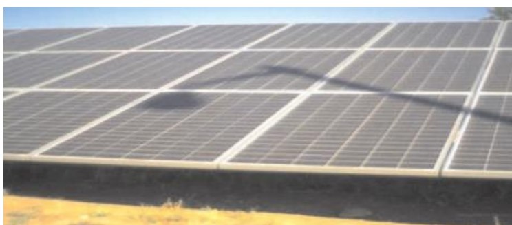
Figure 2.12. Partially shaded PV system by a light pole [92].
