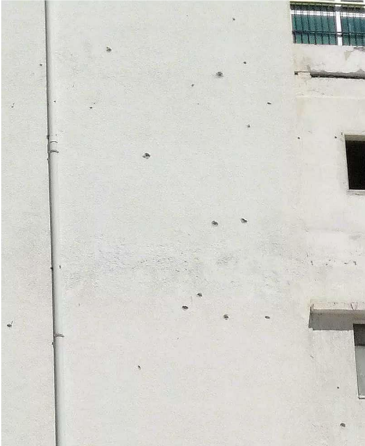
Figure 6.2 Bullet Holes in a Building in Libya
