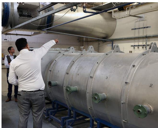
Fig. 5. Commissioning of a 1.5MW unit operating with ammonia blends for steam production. Cardiff University Centre of Excellence on Ammonia Technologies.
