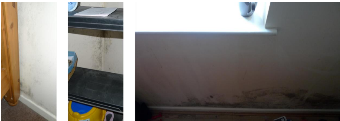
Figure 7-21 Rhondda end-terraced house; pre-retrofit condensation and mould across the west wall.
