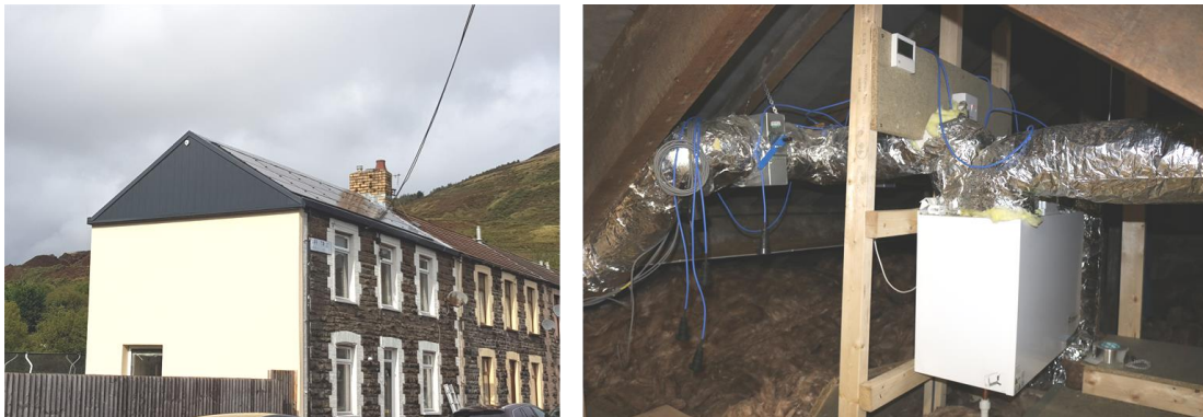
Figure 59. South wall façade integrated TSC (left) and detail of the ducting to the MVHR during construction phase (right) at Rhondda end-terrace house, Wales, UK; author.
