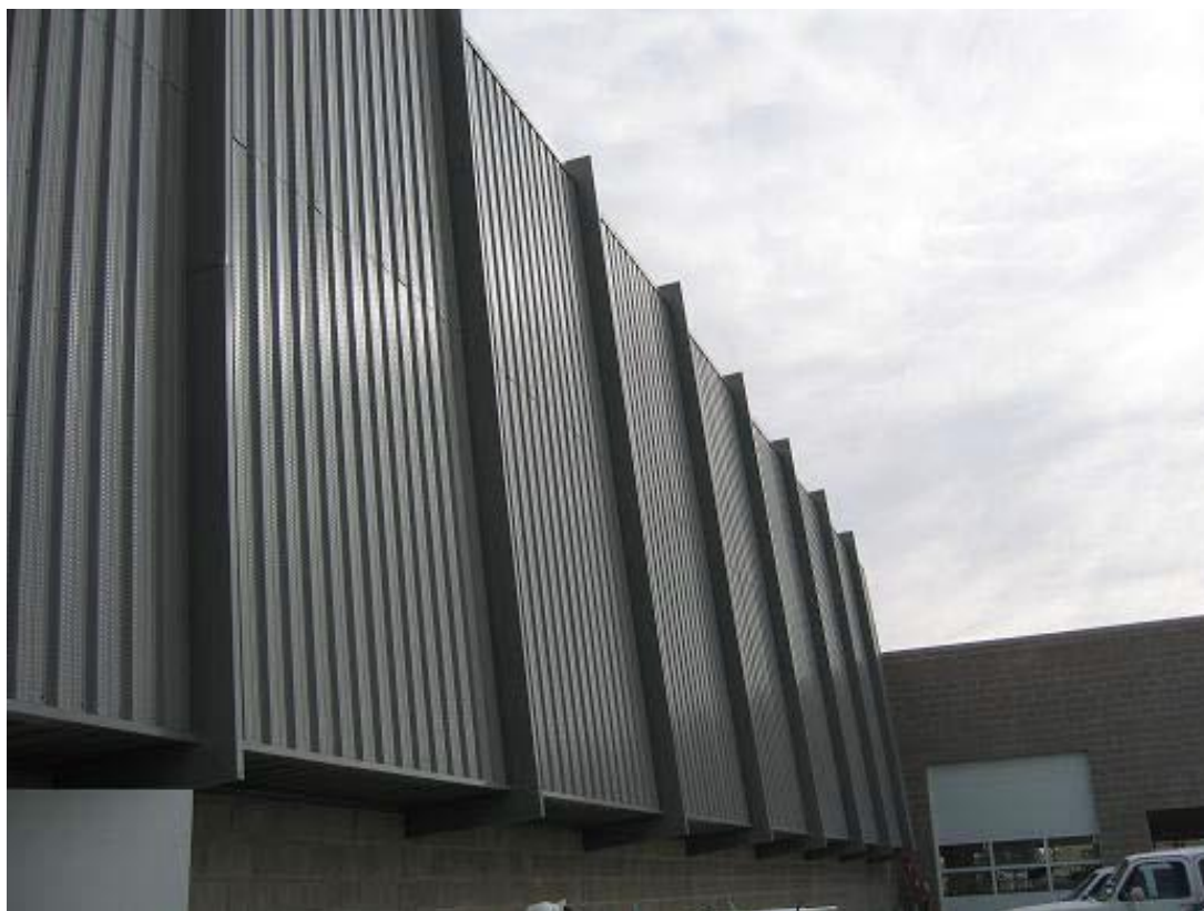
Figure 32. TSC installed on south wall of the Wal-mart store in Colorado (23)
