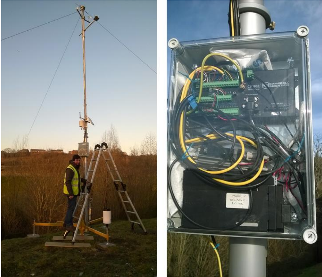
Figure 7-48 SEDA factory. Left: autonomous, solar powered weather station. Right: Waterproof enclosure to accommodate CR1000 logger and battery; author.
