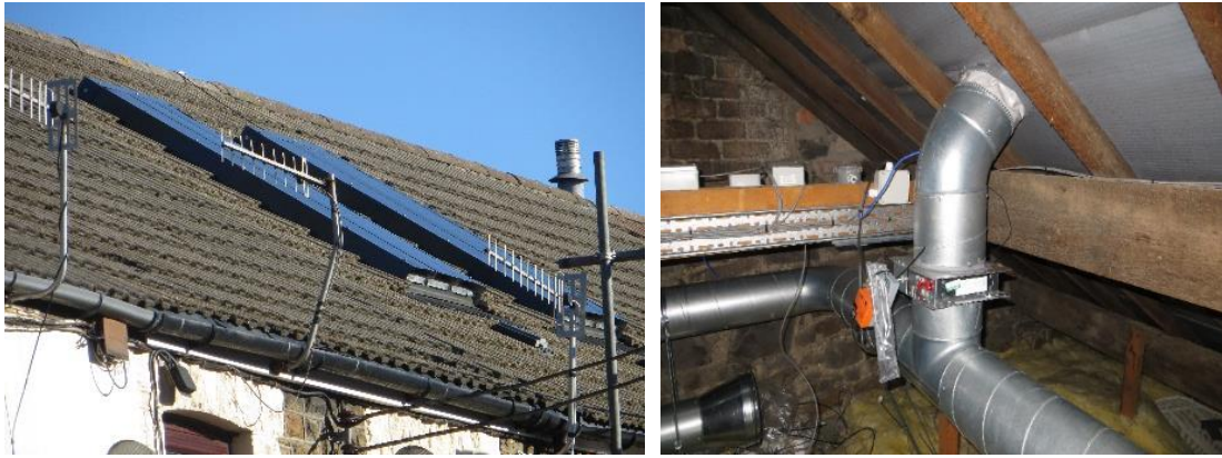
Figure 55. Two small TSCs on an inclined roof (left) and controls and attic ducting (right) at Rhondda terraced house, Wales, UK; author.
