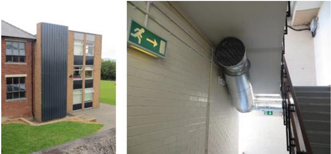
Figure 51. Vertical wall TSC (left) and delivery corridors (right) at Glan Clwyd School, St Asaph, Wales, UK; author.
