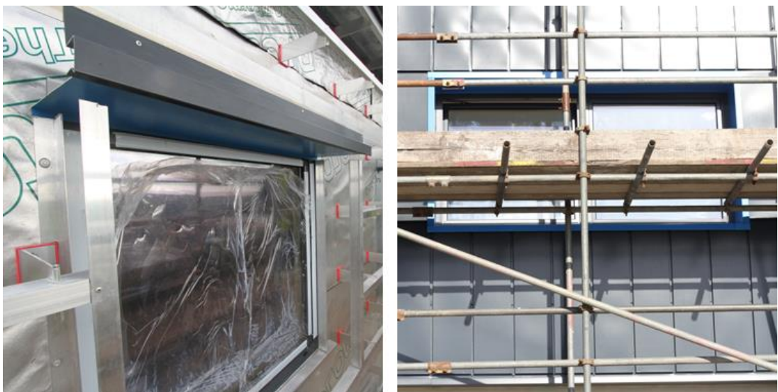
Figure 7-30 Solcer house; TSC supporting structure (left) and end-product (right), LCBE project.
