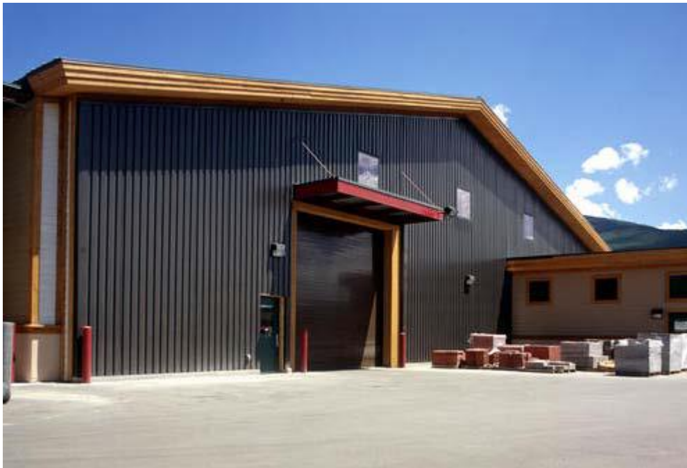
Figure 22. TSC on the south wall of the warehouse (16).
