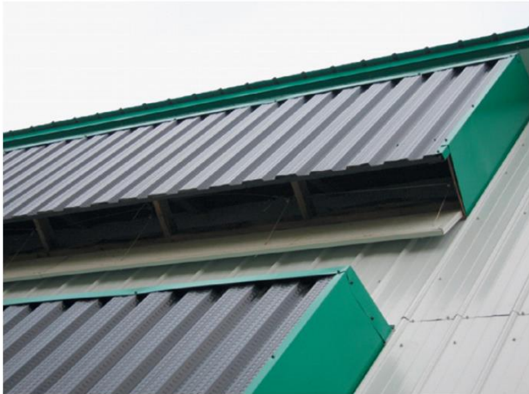
Figure 27. TSCs on the south-east wall of the two broiler barns in Canada, showing the bottom by-pass door (20).
