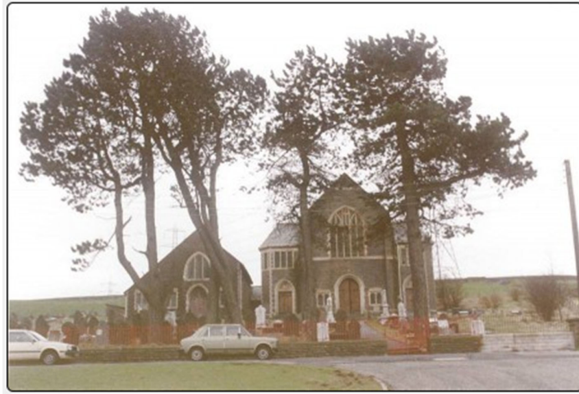
Figure 21 Onllwyn Chapel before demolition. Note the tower to the side had already been demolished at this time (Source: Cwm Dulais Historical Society )
