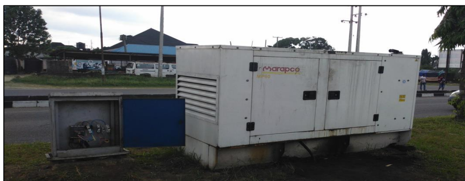
Fig. 3.14. Diesel generator output to AC Panel used for municipal street lighting.
