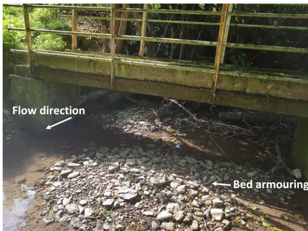
Figure 5.22: Downstream of dam 28 in the mid reach illustrating armouring of the bed. The presence of an armoured layer on the bed surface is quite a common phenomenon which increases the roughness of the bed surface downstream of the WDD. Photograph taken: 19 th Sept. 2020.
