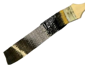
Figure 31 Application of modified epoxy on CFRP sheet before installation on to the concrete surface.
