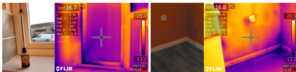
Figure 6: Thermographic imaging results (above: window frame; below: skirting board)
