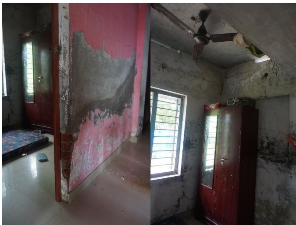
Figure 8.5: Condition of one of the houses in East Manjanakkad Island after the flood in 2018.
