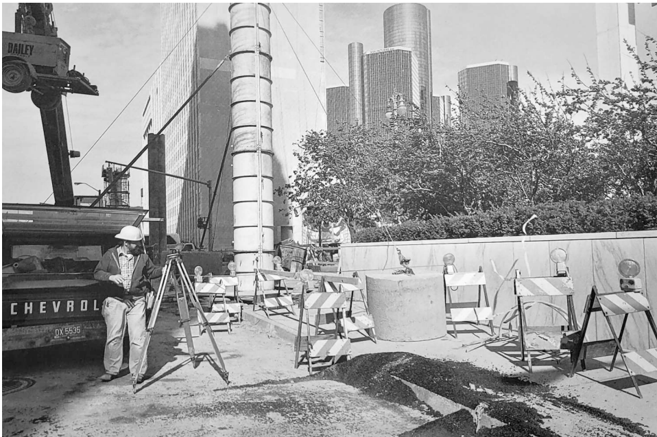
Figure 4. Downtown People Mover construction with towers of Renaissance Center at right rear, Larner west of Woodward facing east, May 24, 1984, photographer Douglas Aikenhead. Source: Courtesy of Aikenhead
