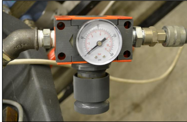
Figure 3.2.5 The regulator in place on the air line.
