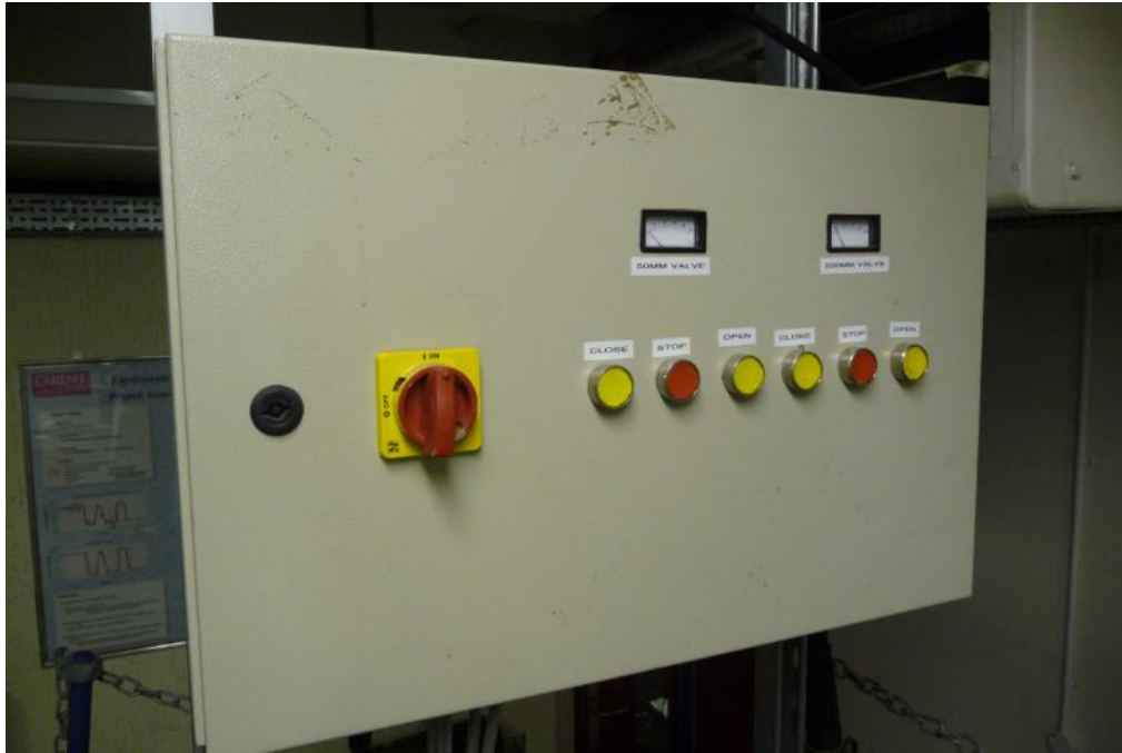
Figure 3.2 Valve control panel
