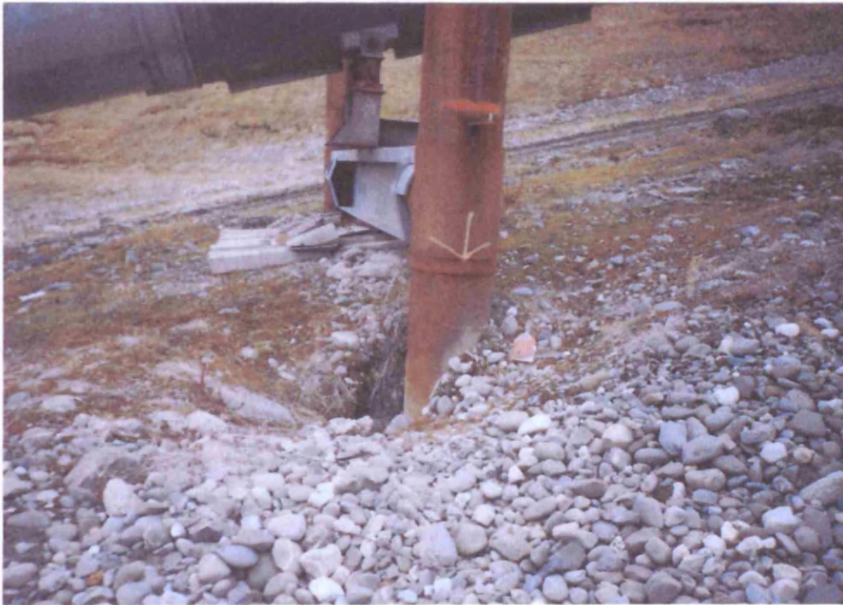
Figure 1.3.2. Active-layer solifluction around vertical pile supports for the Trans Alaska Pipeline System (TAPS), Alaska, USA. The vertical support members are embedded in permafrost, and near-surface solifluction has caused significant distortion of the pile. (Photograph: R. G. Tart).
