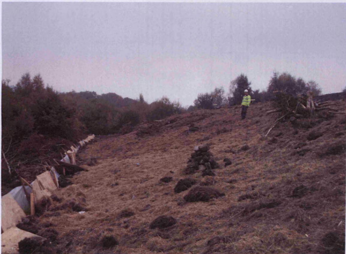
Figure A4.6 The finished enhanced site showing both hibernacula (to the right of the author), stone and log piles and arisings distributed across the site.
