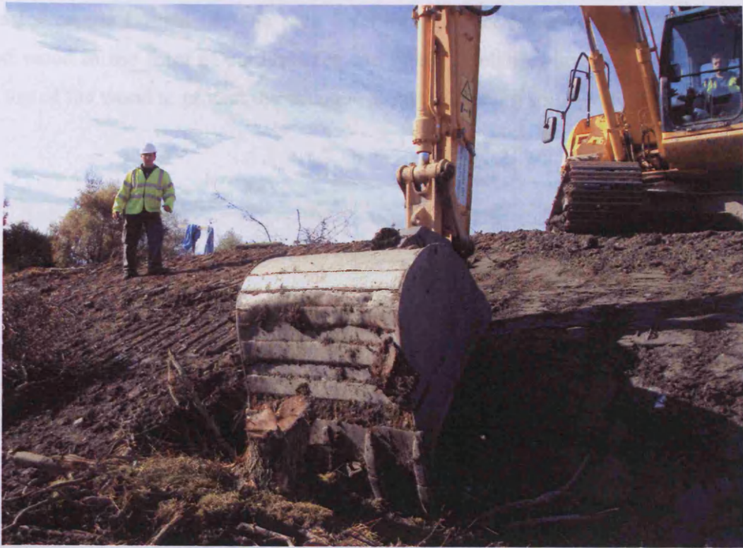
Figure A4.2 The author directs the placement of tree roots at the south facing edge of the hibernacula entrance.
