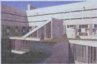
Figure 107. Green roofs at the courtyard of Le Corbusier’s Monastery of La Tourette (Baker, 1996)
