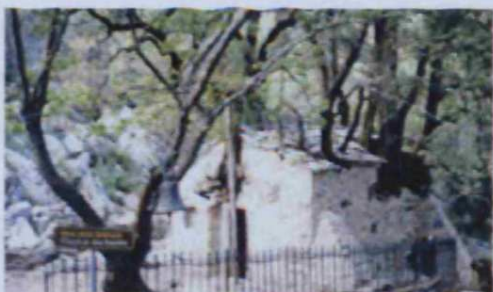
Figure 50. View of the church of Ayia Theodora, with trees on its roof (University of Patras, 2001)
