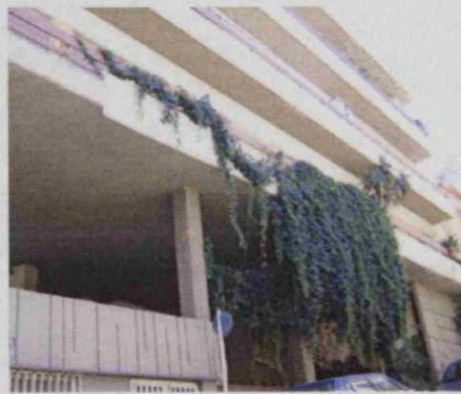
Figure 43. Green curtains hanging in the entrance of a building apartment in Athens (author)
