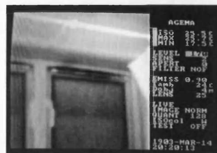
Figure 116: Thermography Survey – Lounge Open Trickle Vents
