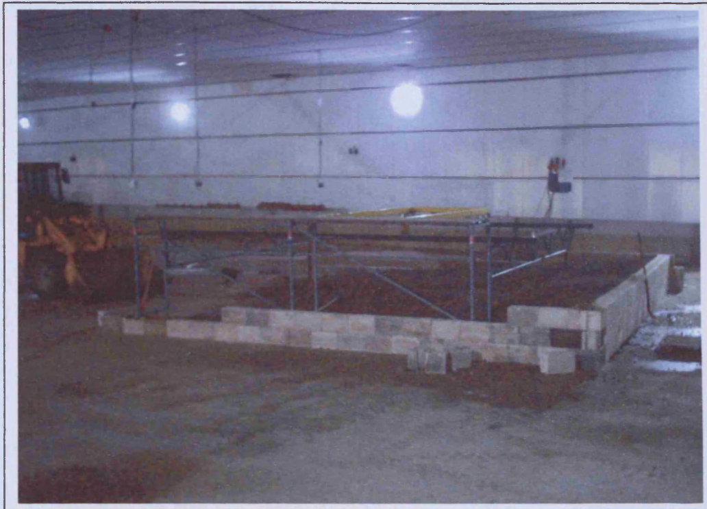
Figure 7.2.2: Details of the boundary in the rear side of the experimental beach
