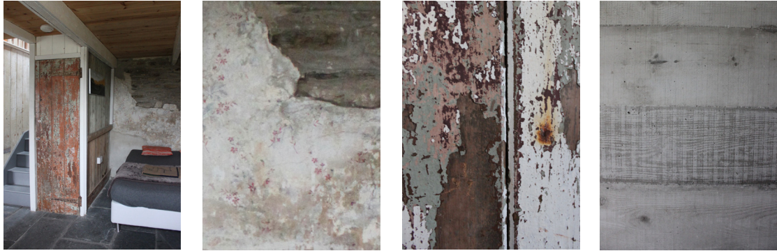
Fig. 7.12 Contrasting textures of interior; Fig. 7.13 Wall paintings on plasterwork covering exposed stonework in places; Fig. 7.14 Layers of paint left on the wooden walls of the staircase; Fig. 7.15 Textured board marked concrete of new extension
