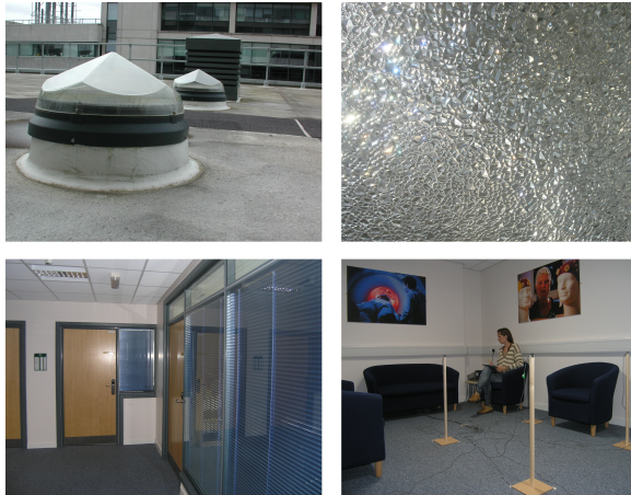
Figure 10 (Top left) Sky-tube, top dome detail. (Top right) Ceiling diffuser. (Bottom left) View of room separator with interior blinds. (Bottom right) Installation with sensors and the person’s position.
