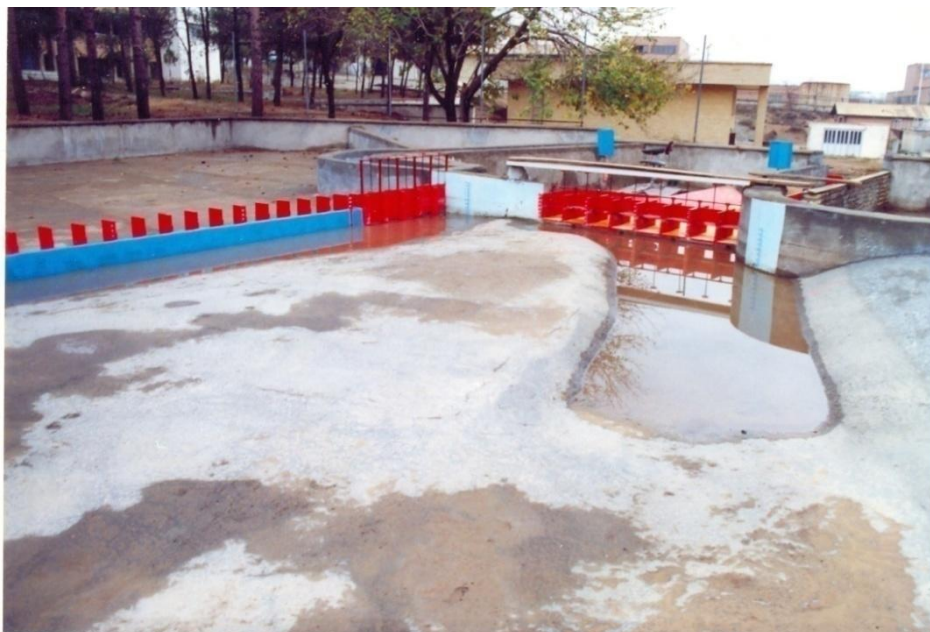
Figure 3.26 The dredging zone in front of Azadegan intake before running the sediment transport scenarios
