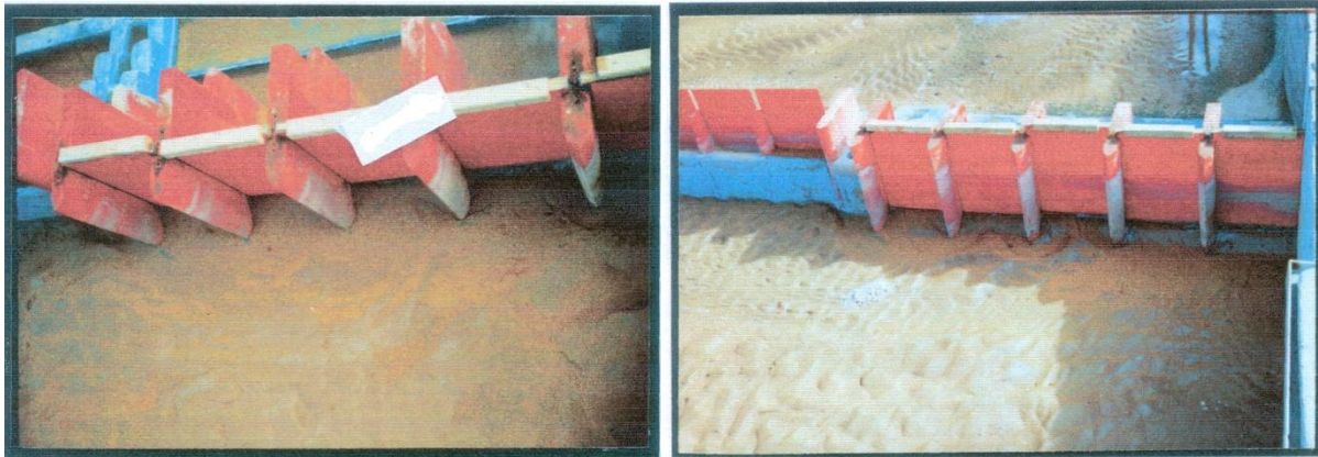
Figure 3.28 Scour zone in front of the right sluice gates
