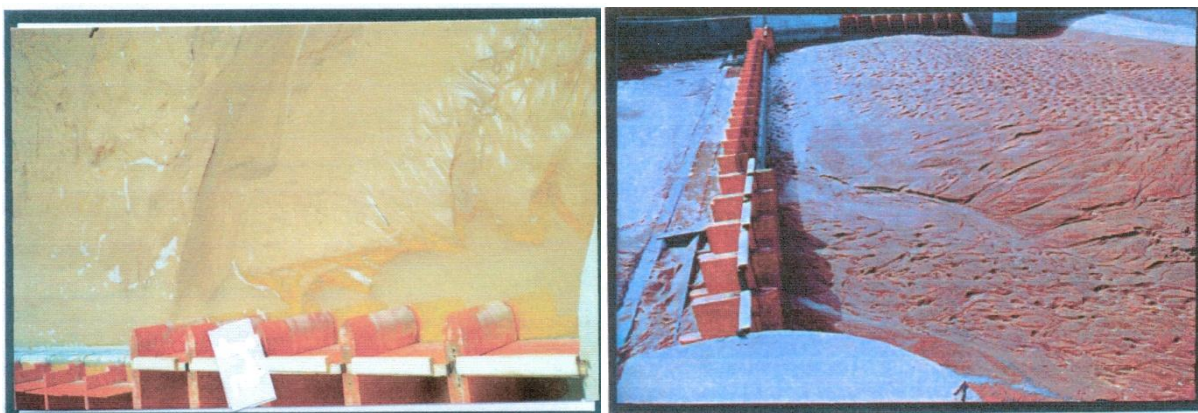
Figure 3.29 Scouring zone in front of the left side sluice gates
