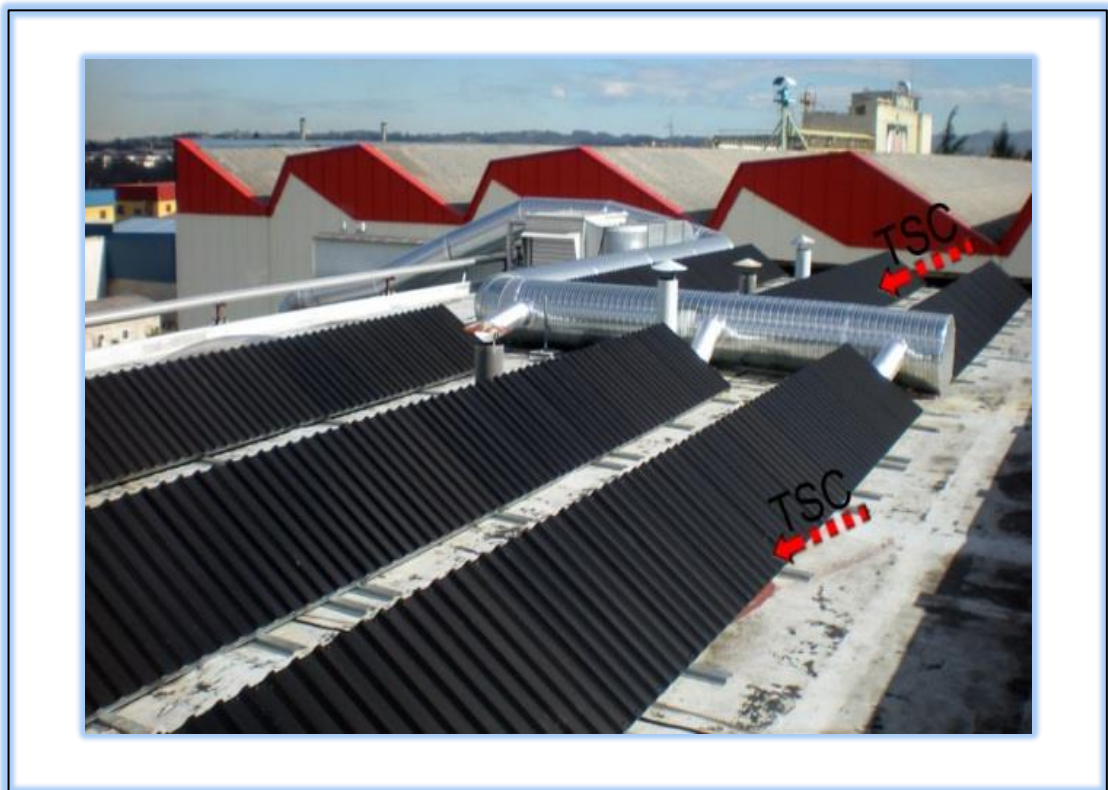
Figure 5-25: Roof integration – TSC duct, (Rena), Renault dealership, Spain (SolarWall n.d.)
