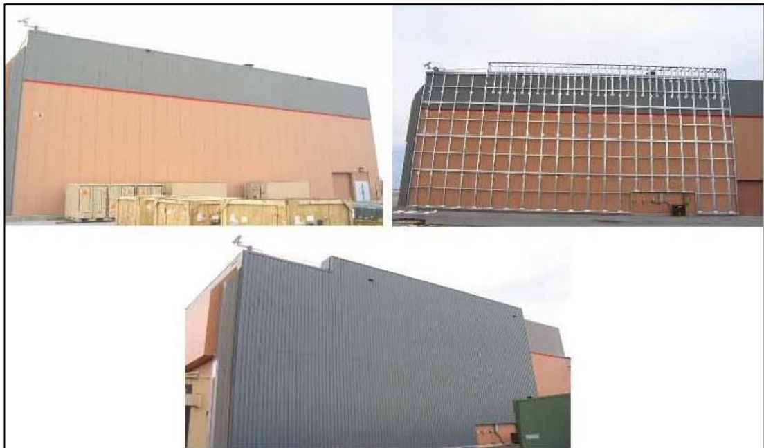
Figure 2-11: Before, supporting framing, and after installation of TSC (Rowley 2007, cited in Brown 2009)
