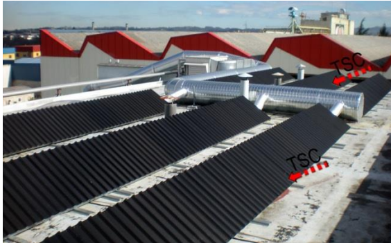
Roof integration – TSC duct, (Non-domestic Commercial Building). Renault dealership, Spain (Solarwall, n.d)
