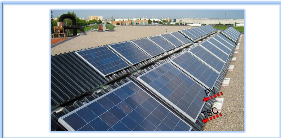
Figure 5-27: Roof integration – PV/TSC (Turn). Turner Fenton School, Ontario - Canada, (SolarWall n.d.)
