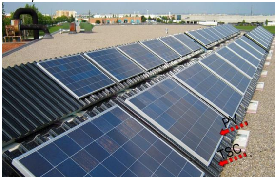
Roof integration – PV/TSC (Non-domestic Institutional Building). Turner Fenton School, Ontario - Canada, (Solarwall, n.d)
