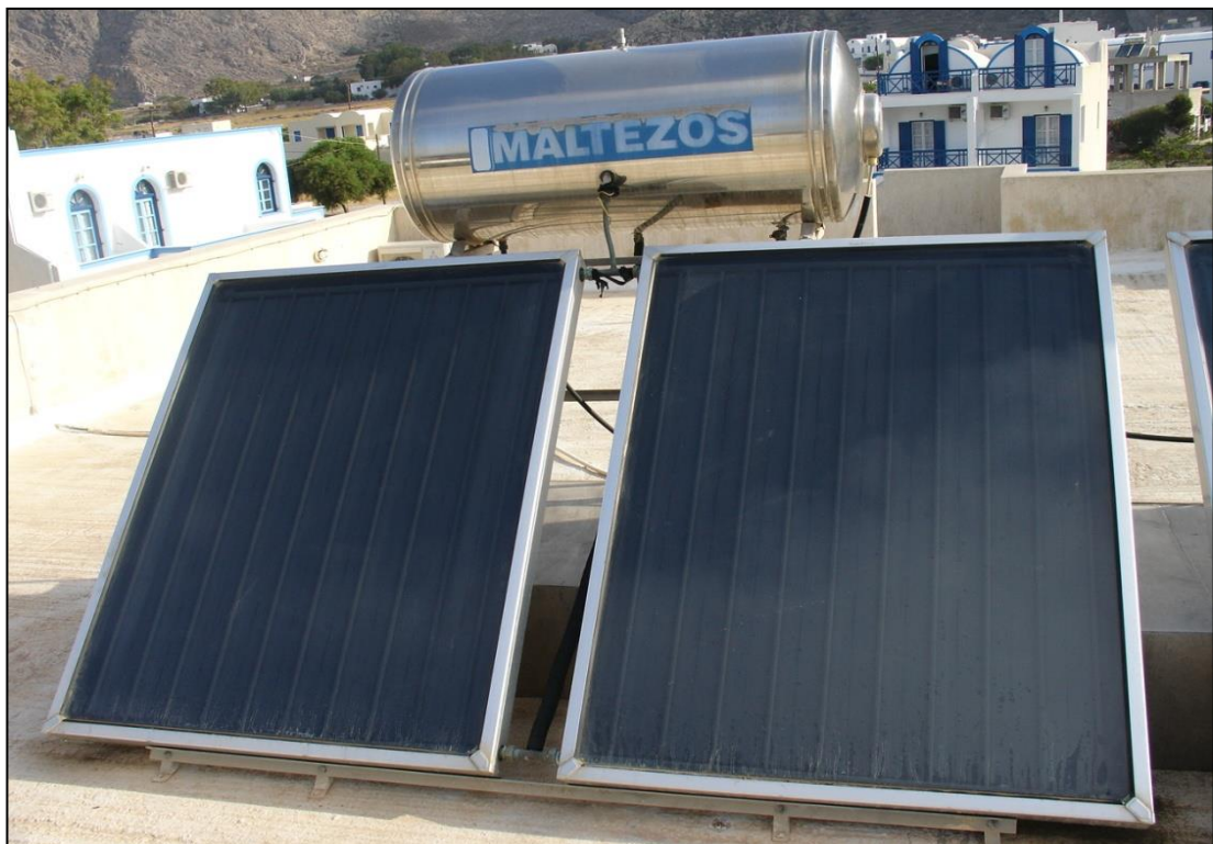
Figure 2-5: Flat-plate thermal system for water heating deployed on a flat roof (Qwiki 2011)
