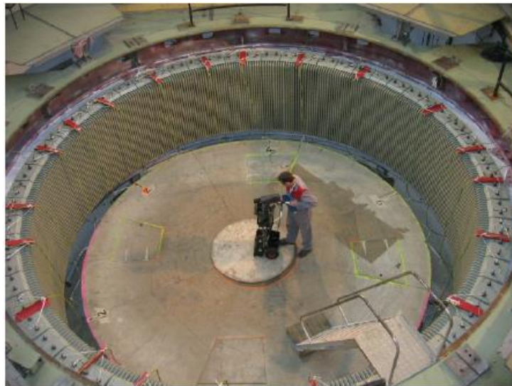
Fig 3-14 Hydro generator core ring flux test using infrared camera for core temperature monitoring [3.9]
