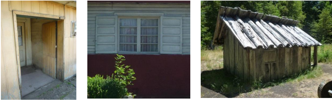
Fig. 1. Double door, Curacautin. Fig. 2. Shutters, Curacautin. Fig. 3 Interlocking timber cladding, Casa del Colono, Conguillio
