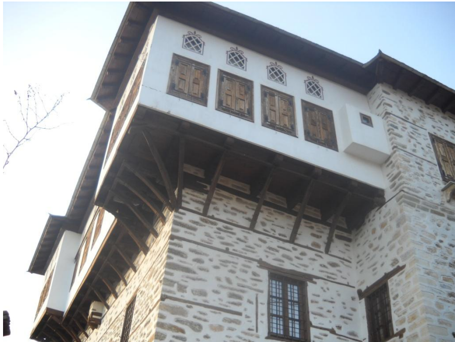
Figure 40: The extension of the top floor supported by woods (sahnisia: σαχνησιά) in mansion house in Agios Lavrentios
