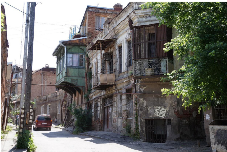
Fig. 15. Dilapidating historic buildings in Old Tbilisi. Photo by Oleg Golubchikov.
