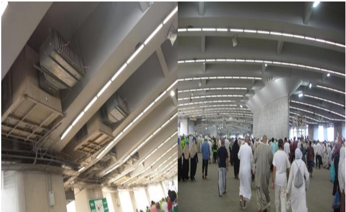
Figure 7-15: Air ventilation (researcher's camera 2013).
