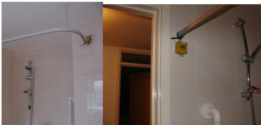
Figure 4.39: temperature and humidity logger next to shower in the bathroom
