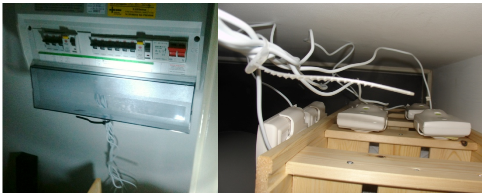
Figure 3.31: Consumer unit and sub-circuit sensors installation
