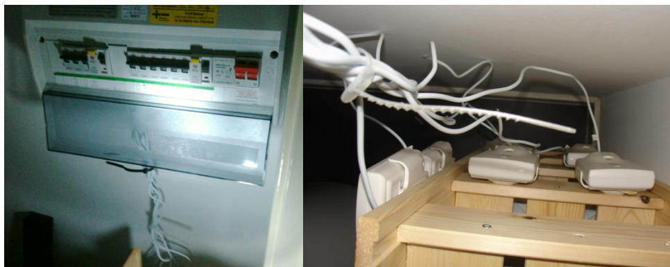
Figure 4.41: Consumer unit and sub-circuit sensors
