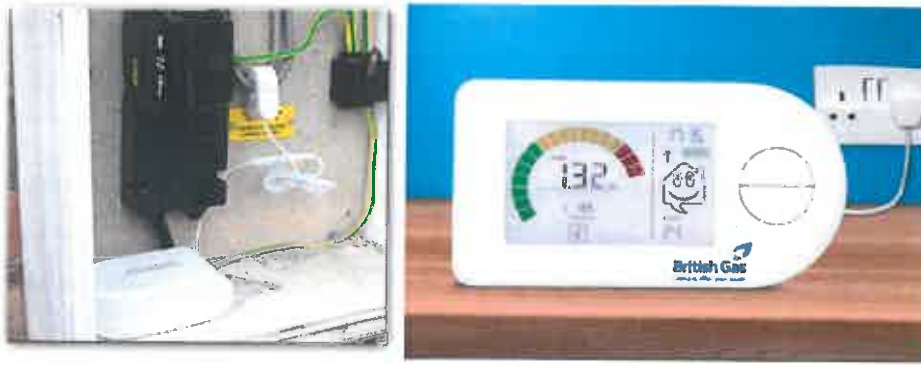
Figure 2.18: Wireless current transducer and electricity monitor, source: author
