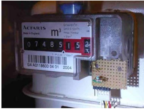
Figure 4.11: Gas meter mounted with optical reader and pulse generator circuit board.
