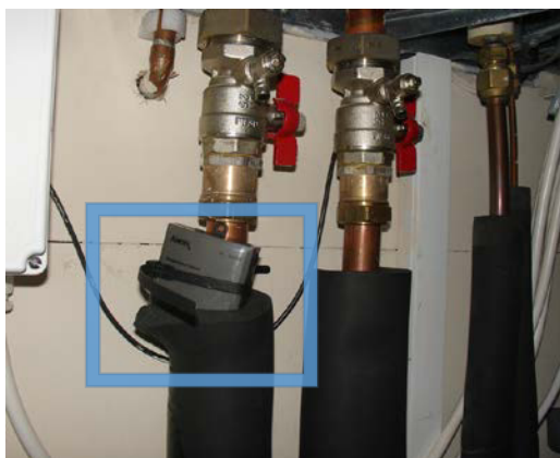
Figure 4.33: Surface temperature sensor on hot water outlet pipe
