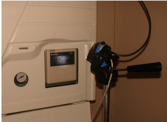
Figure 4.34, infrared camera points at ASHP and immersion heater controller panel
