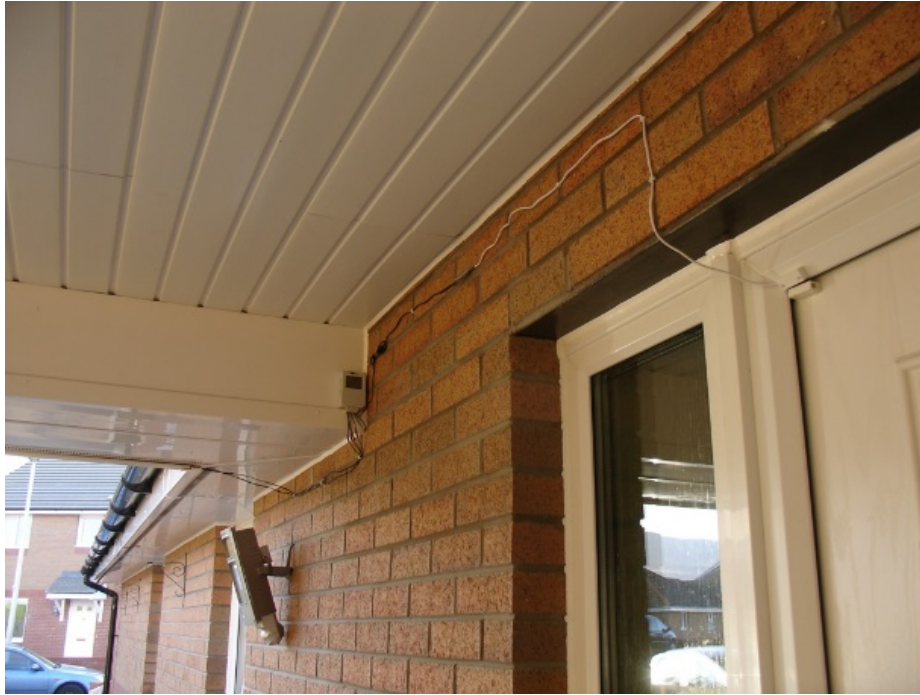
Figure 3.15: contact switch and event logger on a door
