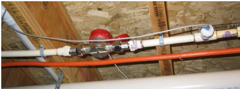
Figure 3.22: Water flow installed in hot water supply pipe.
