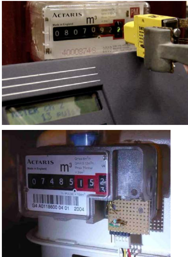
Figure 3.4: Gas meter mounted with infrared reader, optical sensor and pulse counter
