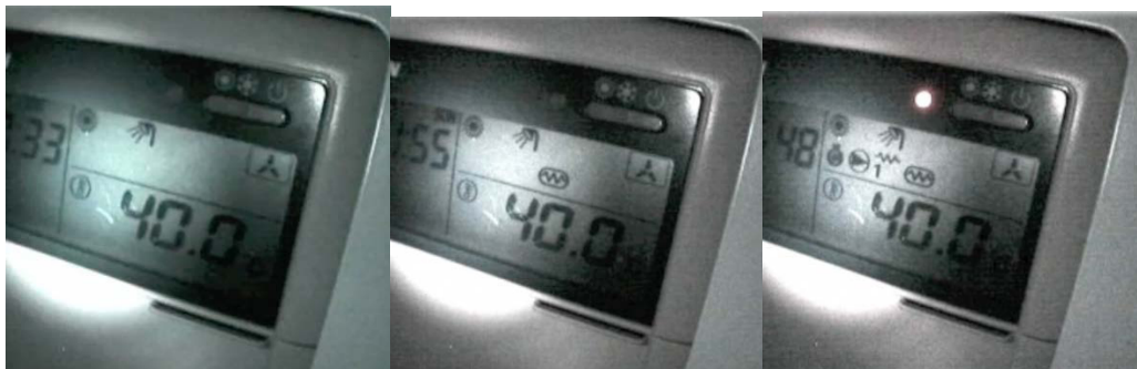
Figure 4.35, Icons for not running, immersion heater running and ASHP running from left to right
