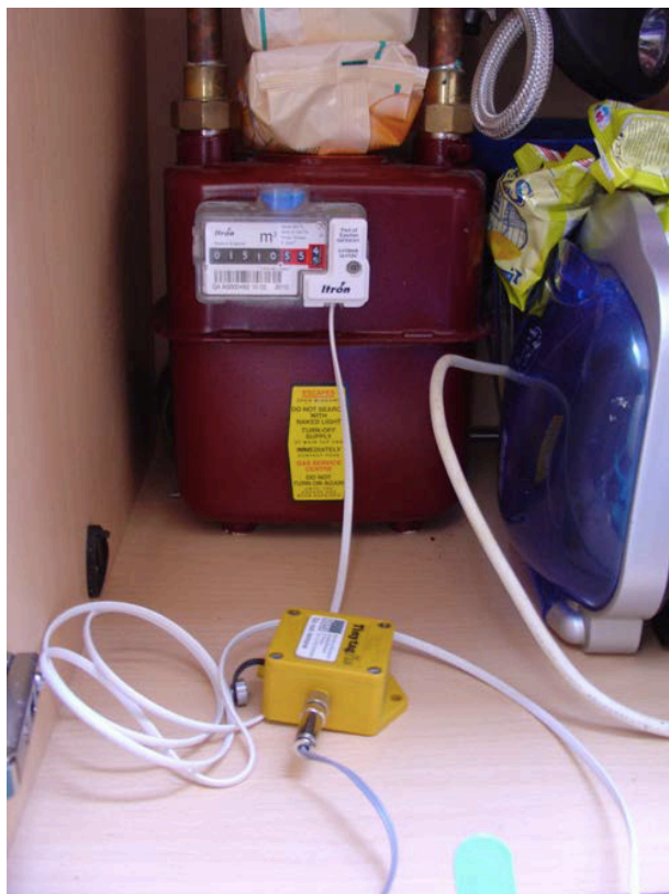
Figure 3.2: G4 gas sub-meter with pulse output and pulse counter logger
