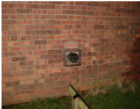
Figure 4.12: Gas fireplace exhaust vent
