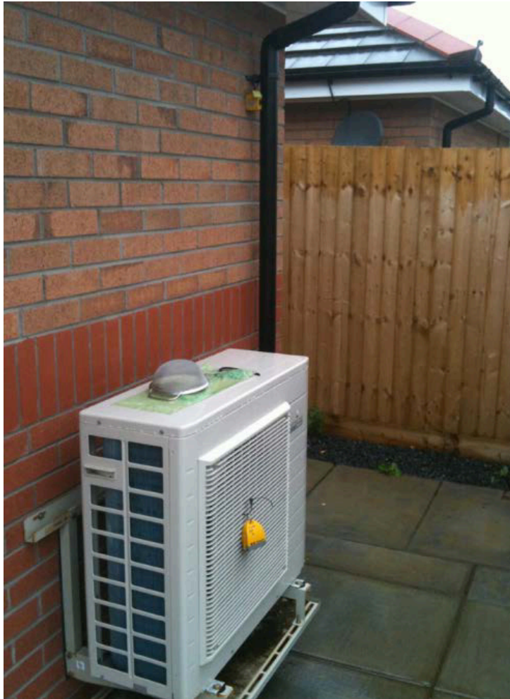
Figure 4.36: temperature on ASHP outdoor unit
