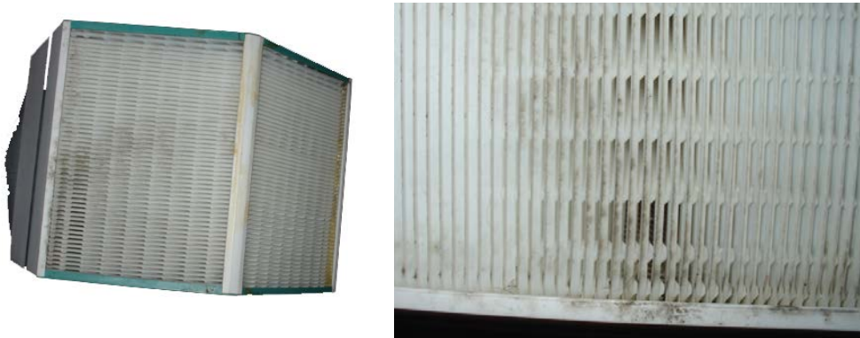
Figure 5.60: Air filter in MVHR system at dwelling 6
