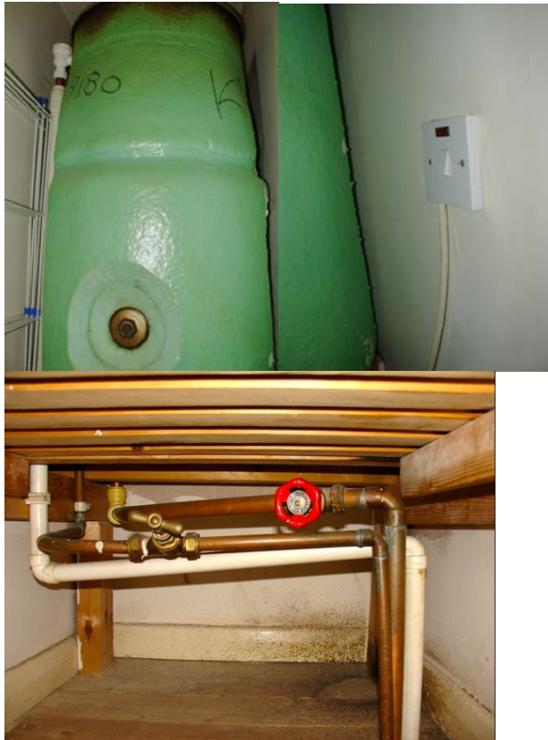
Figure 4.13 Immersion water heater, control switch and hot water outlet pipe underneath
