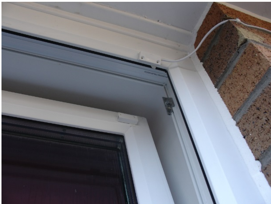
Figure 3.14: contact switch on a window
