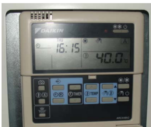
Figure 3.11: Boiler control programmer
