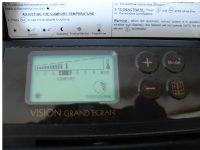
Figure 4.4: Electric radiator control panel
