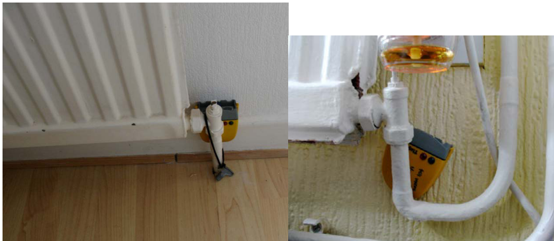
Figure 4.24: Individual radiators and temperature sensor in dwelling 4 & 5
