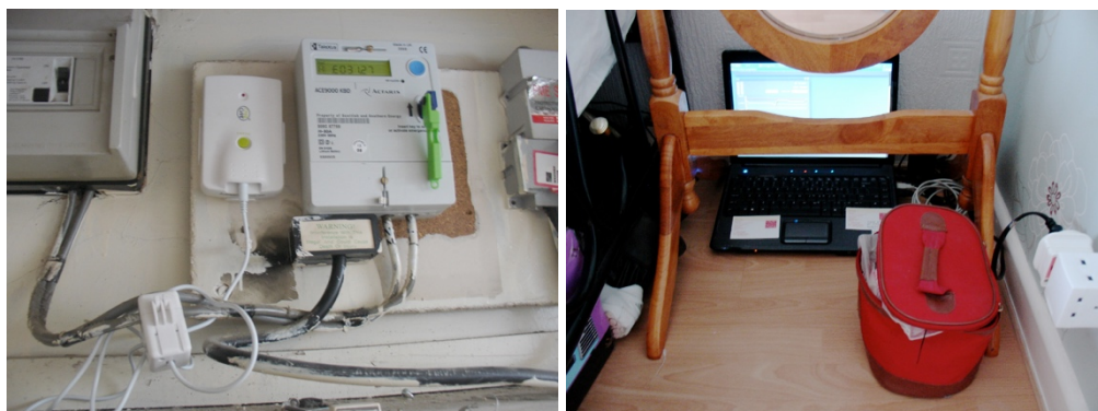
Figure 3.29: Owl energy meter transmitter, receiver and computer set up
