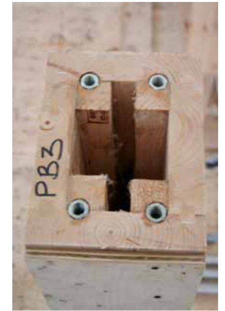
Fig 9.84 Frame and SIPs infill assembly a. The 270x210mm box section posts and beams and SIPs panels were pre coded prior to delivery to match the construction methodology. The box section floor beams and posts were bolted to the steel bearers and each other using end grain bolting. The entire superstructure was assembled in 10 days by a team of 4 carpenters; b. The components were delivered to site in reverse construction sequence, stored in the correct order adjacent to the site and manually lifted into position; c. Completed floor assembly; d. 225mm wall SIPs panels installed with shims to maintain shadow gap around each plywood board; e. 270x210mm box section roof beams are end grain bolted to the posts and used to align the frame; f. Completed frame and SIPs envelope with openings left between posts for windows and doors.
