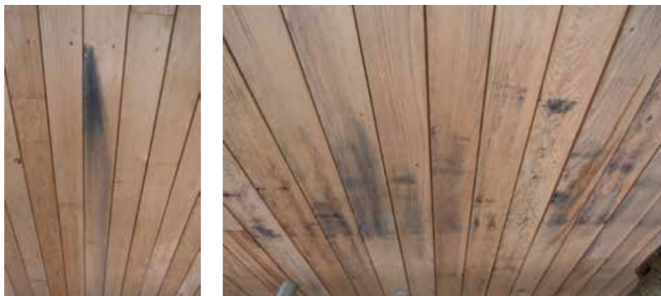
Fig 9.157 Photos of oak cladding stained from interaction with ferrous metals
