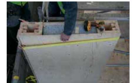
Fig 9.85 Wall assembly details a. Top of post with end grain threaded sockets; b. 225mm thick SIPs walls panel are hand positioned by inserting externally to lap the posts and screwed, providing and internally flush finish between SIPs and frame.
