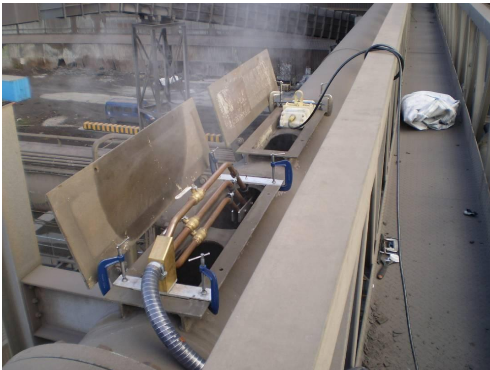
Figure 17: Sampler and flow meter installed in BOS slurry pipe
