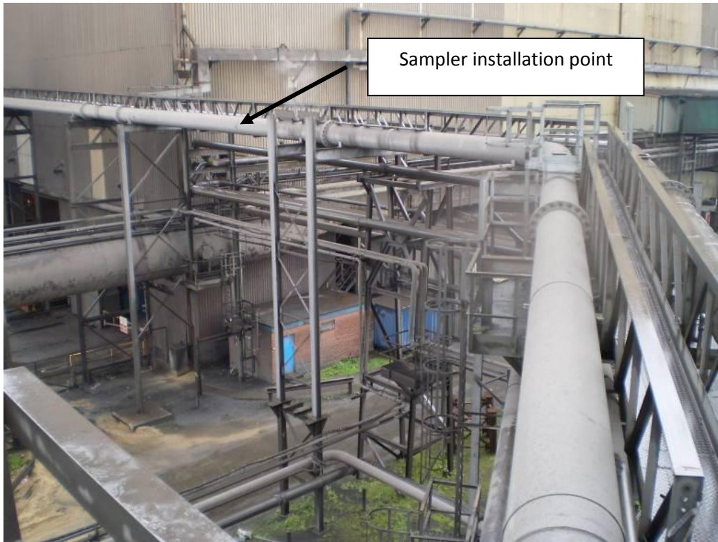
Figure 9: Picture of BOS slurry pipe and sampling point
