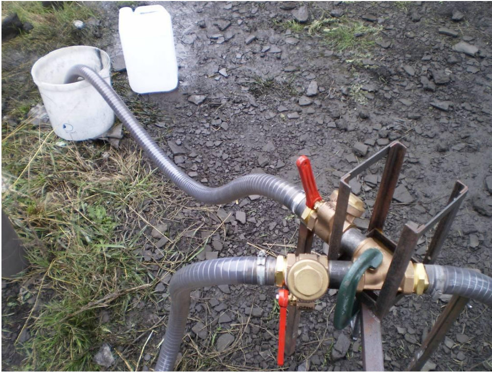
Figure 16: Three way valve at sample point
