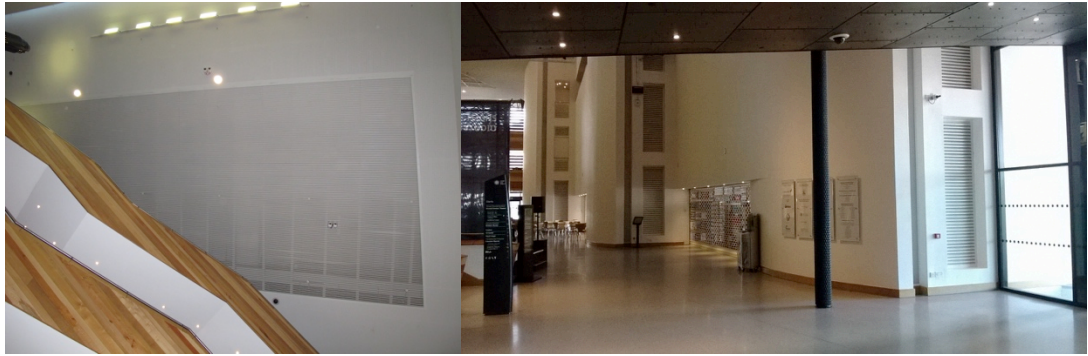
Figure 5.9 Ceiling fans (left) and heat and cool wind outlets (right) in WMC transitional space.
