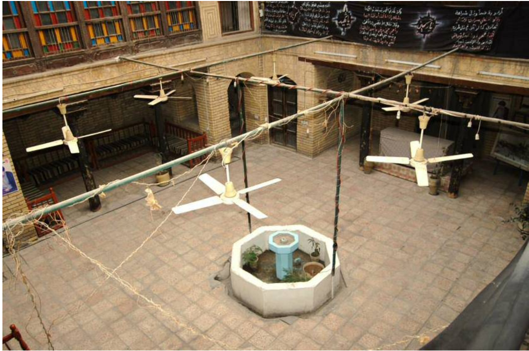
Fig. 4.26. The ceiling fans installed during the dust storms (Researcher)
