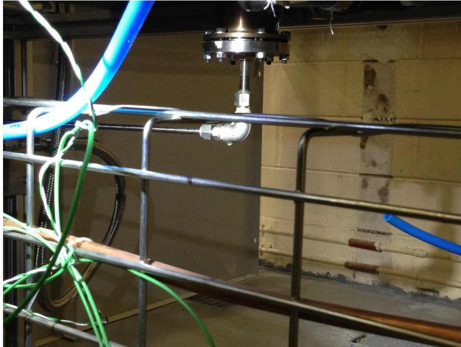
Figure 5-22 Leaking problem in the generic swirl burner
